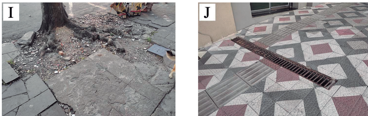
Figure 5 - Damage from vegetation and obstacles on sidewalks.
