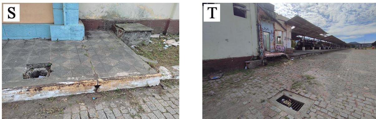
Figure 10 - Lack of accessibility in Railway Station.
